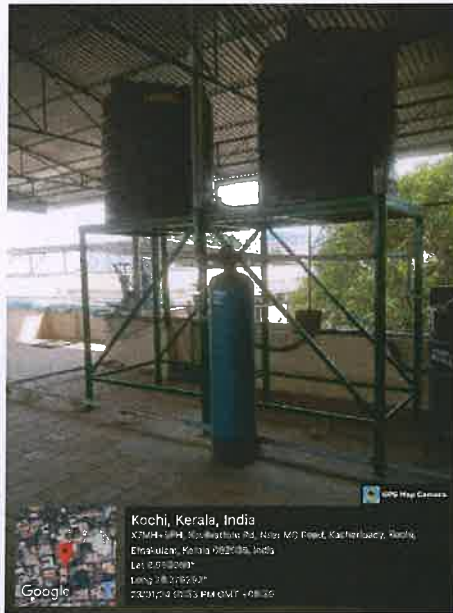
Water Purification System
