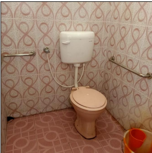
Toilet with Hand Rail
